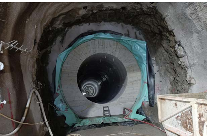
Headrace Power plant Tauernmoos, AT
