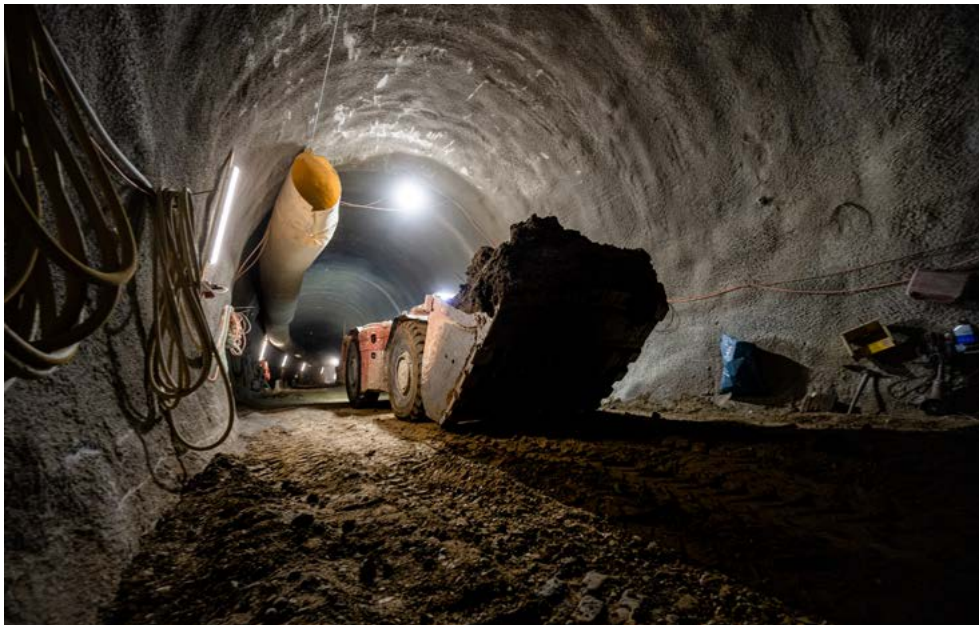
U2XU5, Propulsion track tunnel, Vienna, AT
